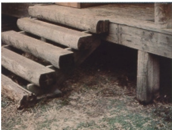
Fig. 17. Wood to ground contact should be avoided at all times. (USFS Photo)
