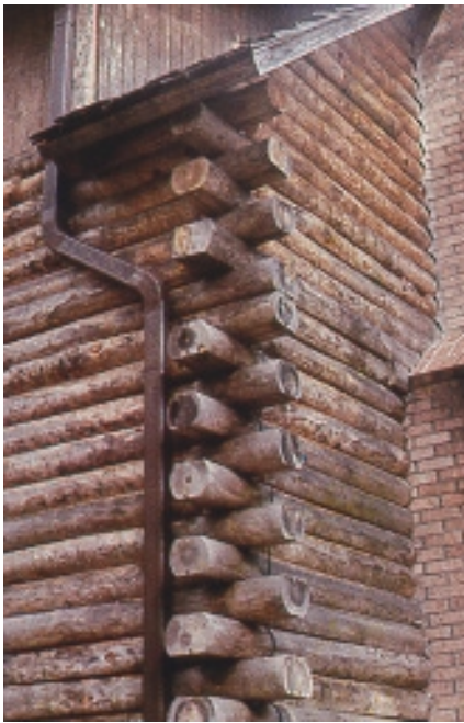
Fig. 4. These log ends are continually exposed to rainwetting. (GFC Photo)
