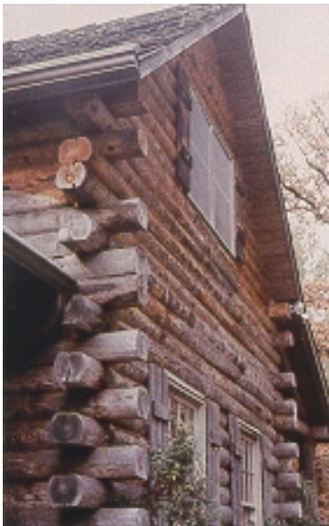
Fig. 3. The logs in this two-story house have been stained from continual rainwetting. Roof overhangs should be at least 24" wide to offer more protection. (GFC Photo)
