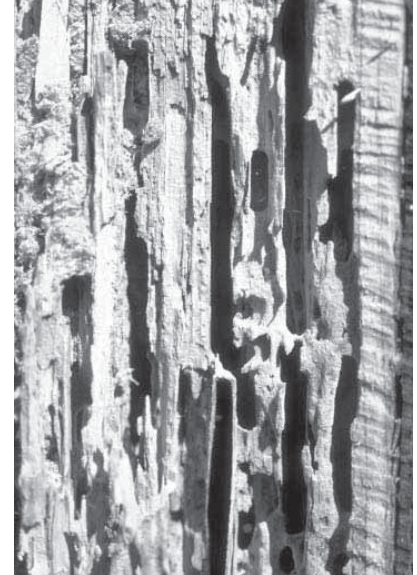
Figure 26B - Carpenter ant galleries
