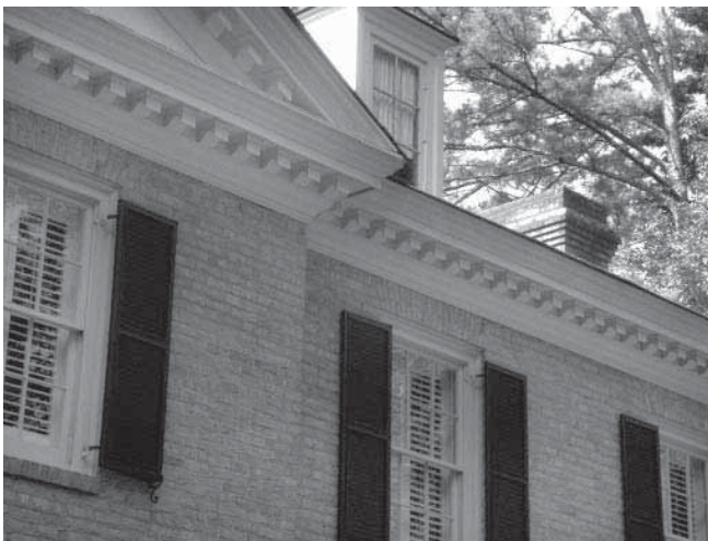
Figure 29 - Carpenter bees readily attack brick and eaves molding
