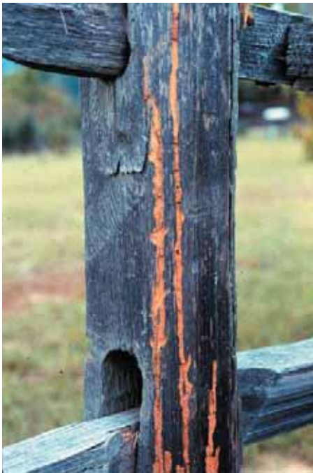
Figure 43 - Termite mud tubes on fence post
