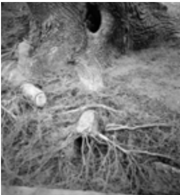
Use of a pneumatic excavation tool combined with a vacuum truck removes soil from tree roots prior to excavation of a curb allowing more roots to be saved.
