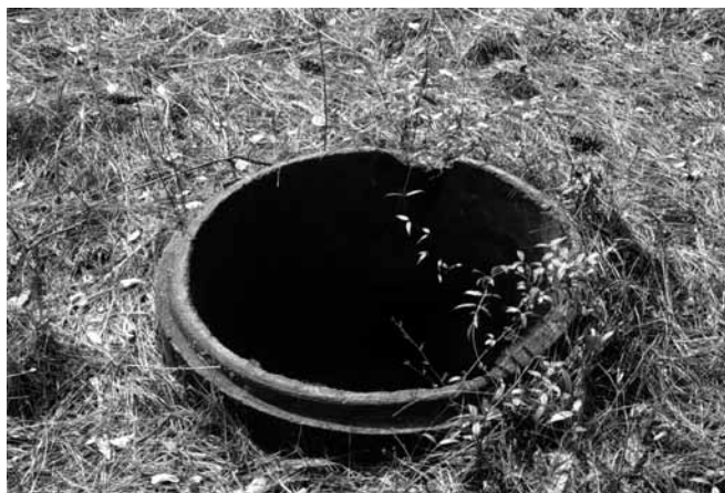
Figure 55 - Abandoned, uncovered water well
