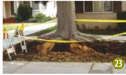
Figure 23 Construction is especially damaging to roots, such as these roots cut during curb repair.
