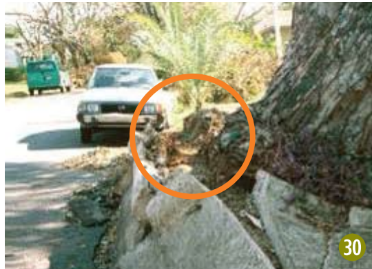
Figure 30 This leaning tree needs to be removed since major structural roots were broken and lifted.
