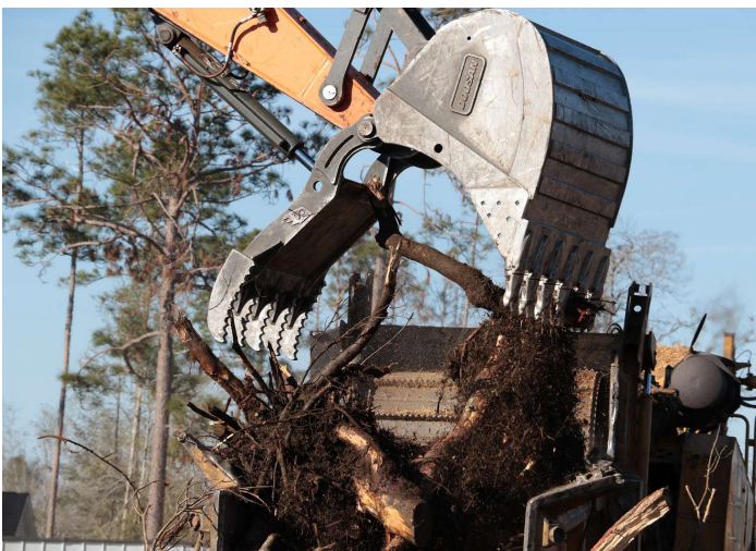
Clean up after Hurricane Michael a 2018 Category 5 storm that brought wind gusts in the 60-75+ mph range to Georgia, downing countless trees and power lines.
